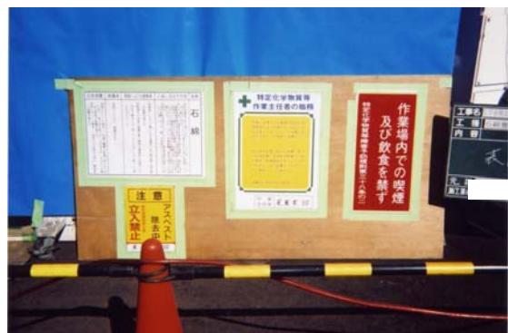
Fig. 12. Signboard for removal of asbestos
