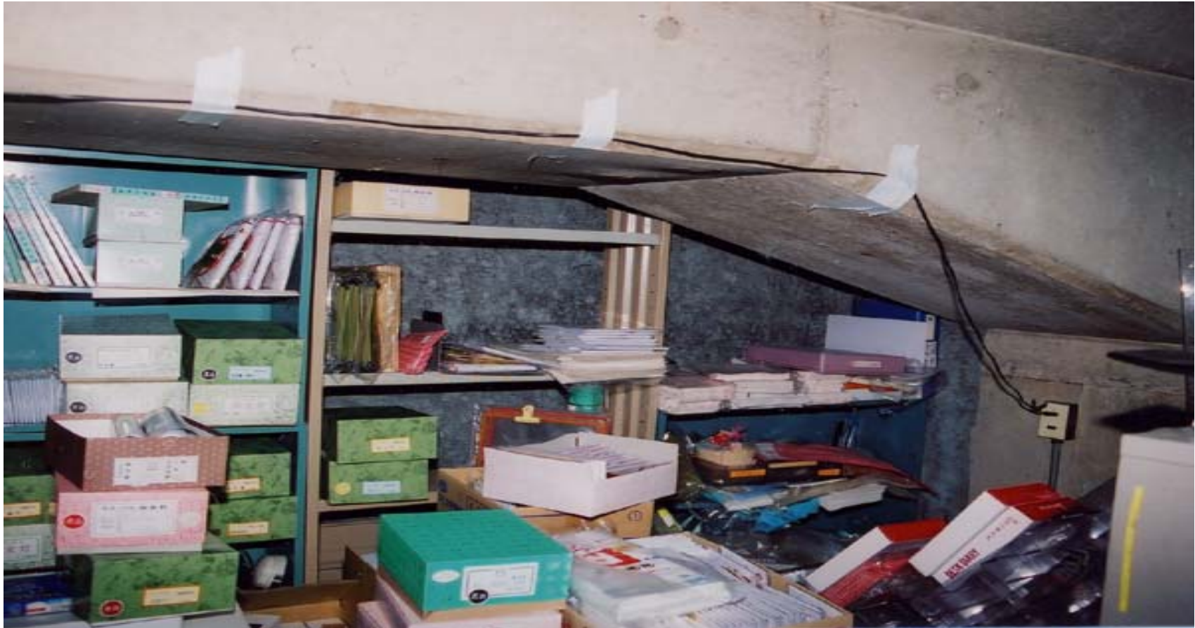
Stationery Store 2nd Floor. Sprayed blue asbestos is on the wall.
