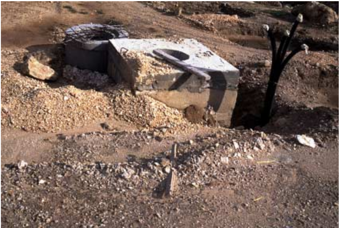
Figure 8. Asbestos debris from excavation on park site. [Full Size]
