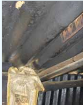
Pitting and smoke damage on AC roofing after long-term use (same dwelling as above).
