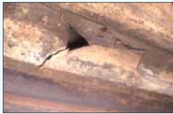
Smoke damaged and cracked AC roofing (same dwelling as above).
