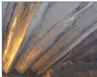
Charred and cracked AC roofing after long-term use (same dwelling as above).
