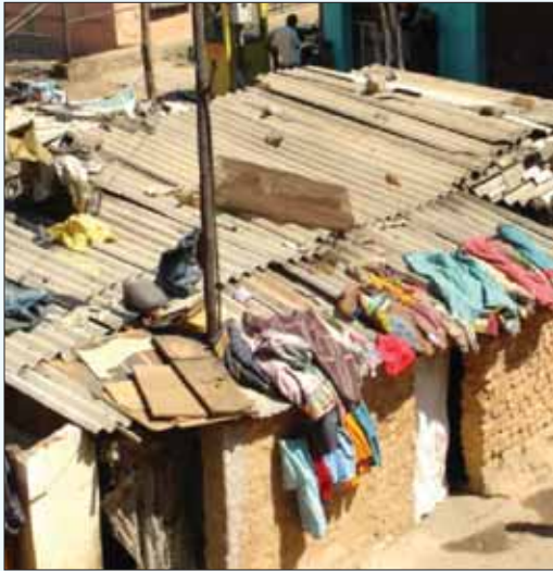
Typical AC roofing in New Lingarajapuram, Bangalore. Note lack of ventilation apart from that available by using the doorway.
