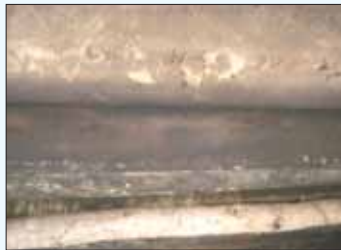
Flaking and pitted AC roofing, resulting from smoke damage. House was newly built and had been occupied for one year at the time of survey.
