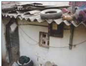
Typical exterior condition of AC roofing in New Lingarajapuram. Note the broken AC roofing sheets, low roof height and the ventilation 'window' – a typical size in the homes of New Lingarajapuram.
