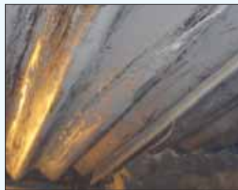
Charred and cracked AC roofing after long-term use (same dwelling as above).
