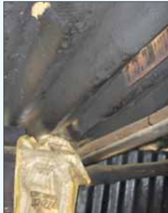
Pitting and smoke damage on AC roofing after long-term use (same dwelling as above).
